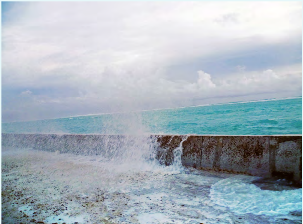
Flooding over seawall
